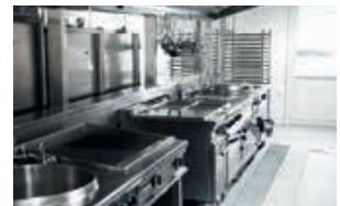
Large-scale catering facilities
