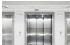
Lifts and elevators
